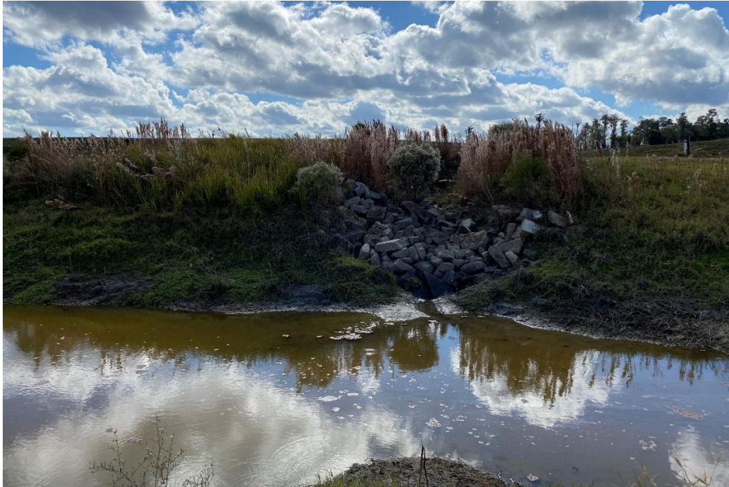
Figure 8. Thick Vegetation Around the Culverts Located on the North Side of Cell 3
