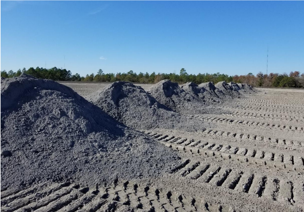
Figure 10. Several Loose Piles on Top of Landfill
