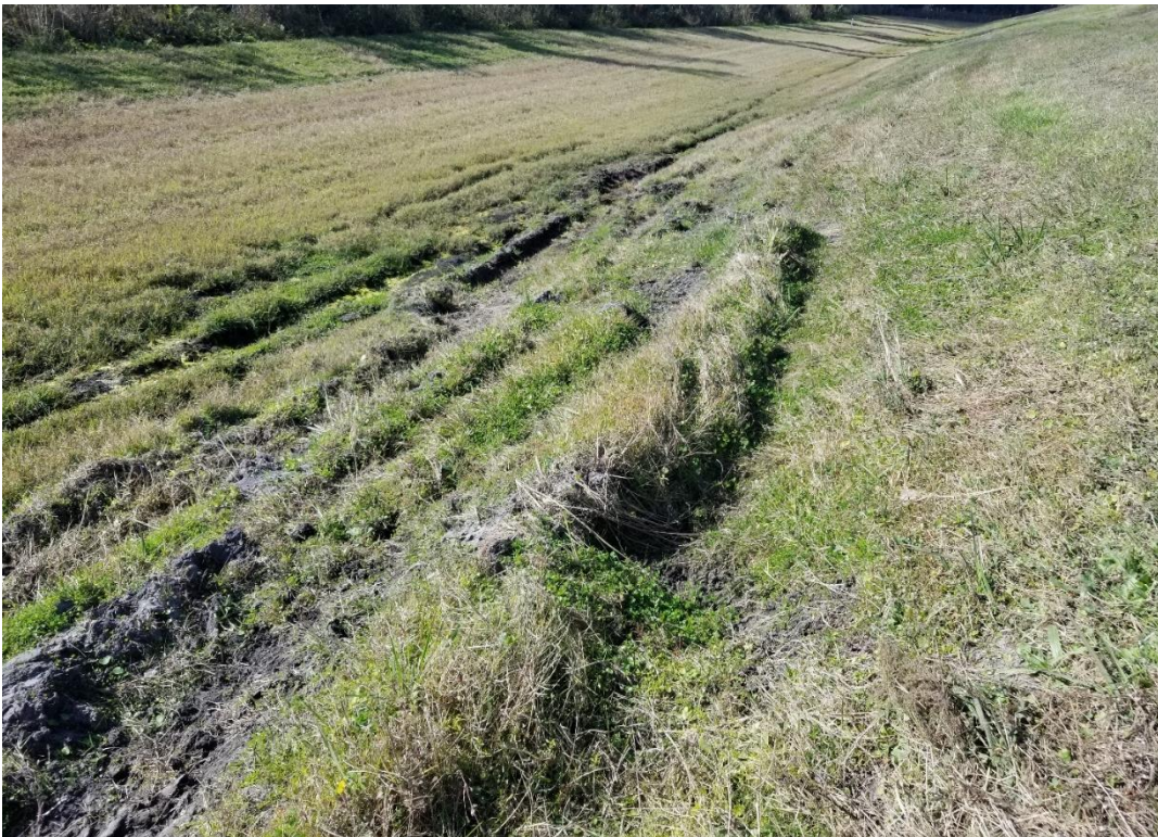
Figure 7. Erosion on Southeast Corner on Landfill
